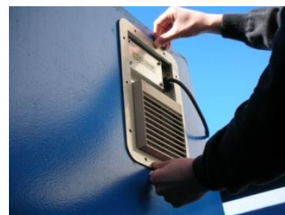
Installation i sopkomprimator
